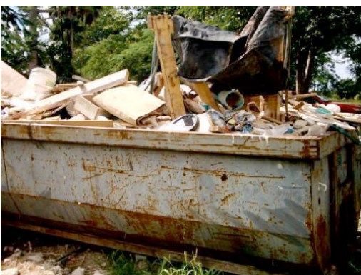
Unacceptable use of dumpster
